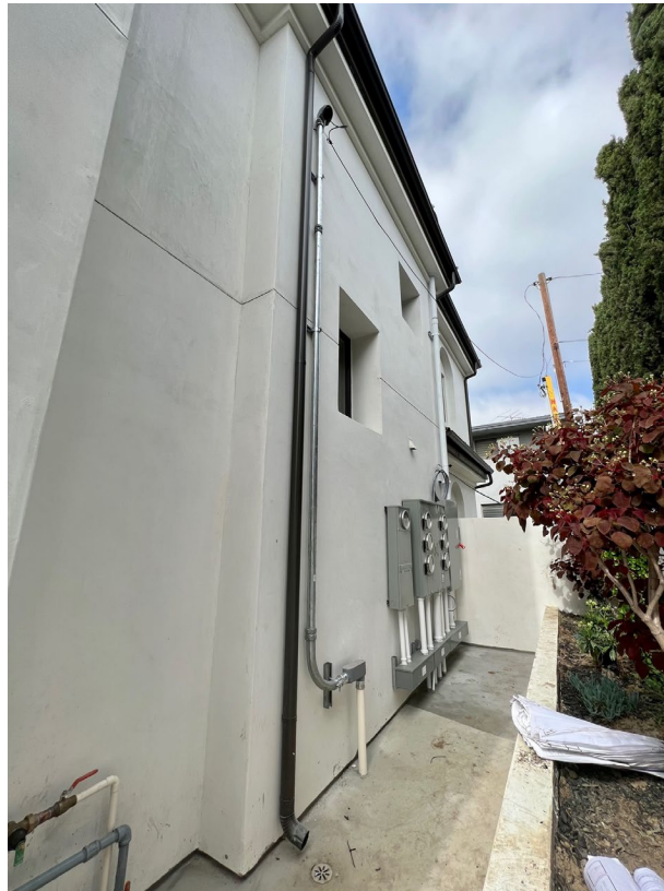
Figure 2 – The rear of the building as constructed showing the rear block wall (right), and the electrical panels on the building
