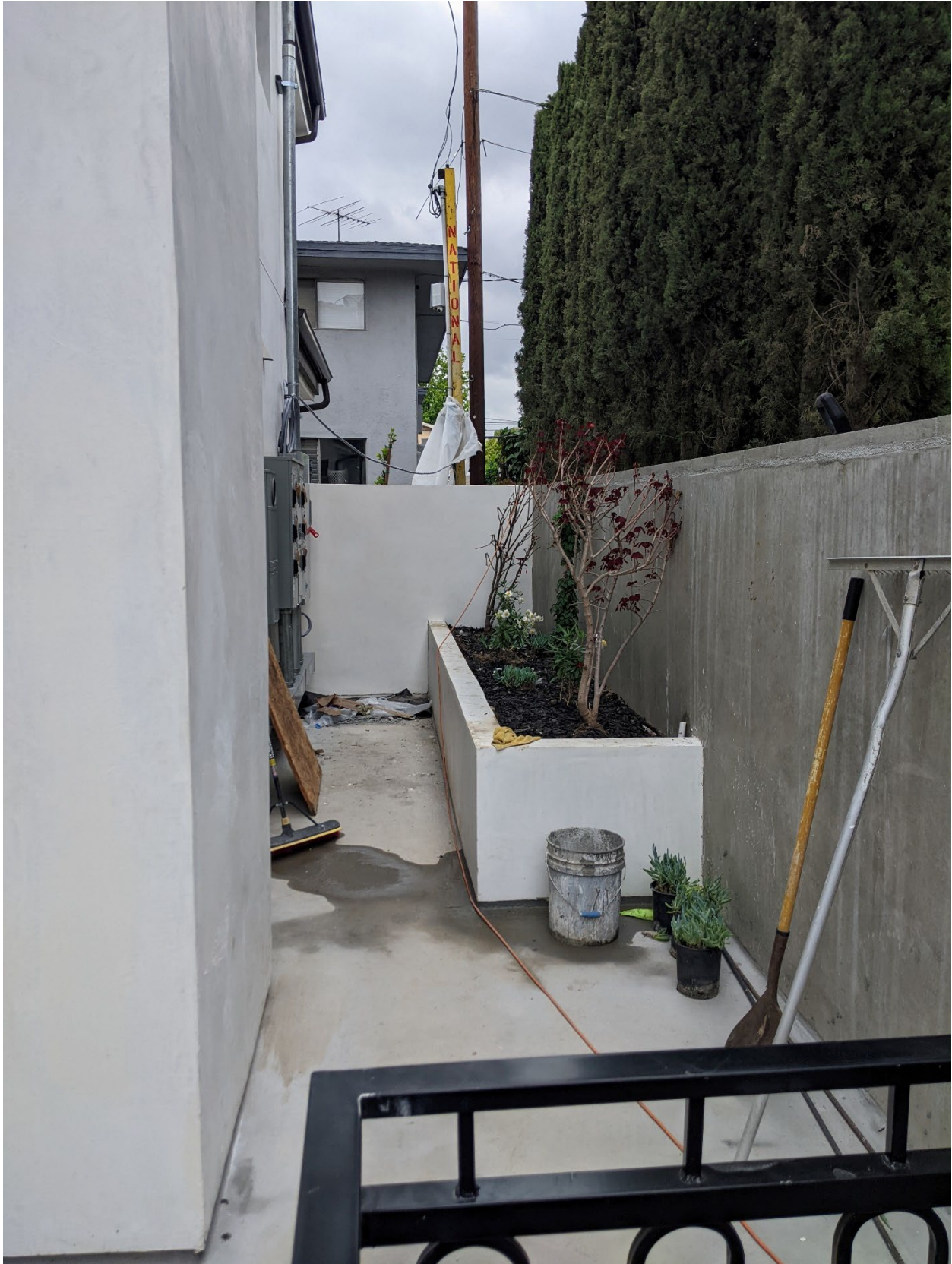
The rear yard of the subject property showing the non-conforming setback and the electrical panel.
